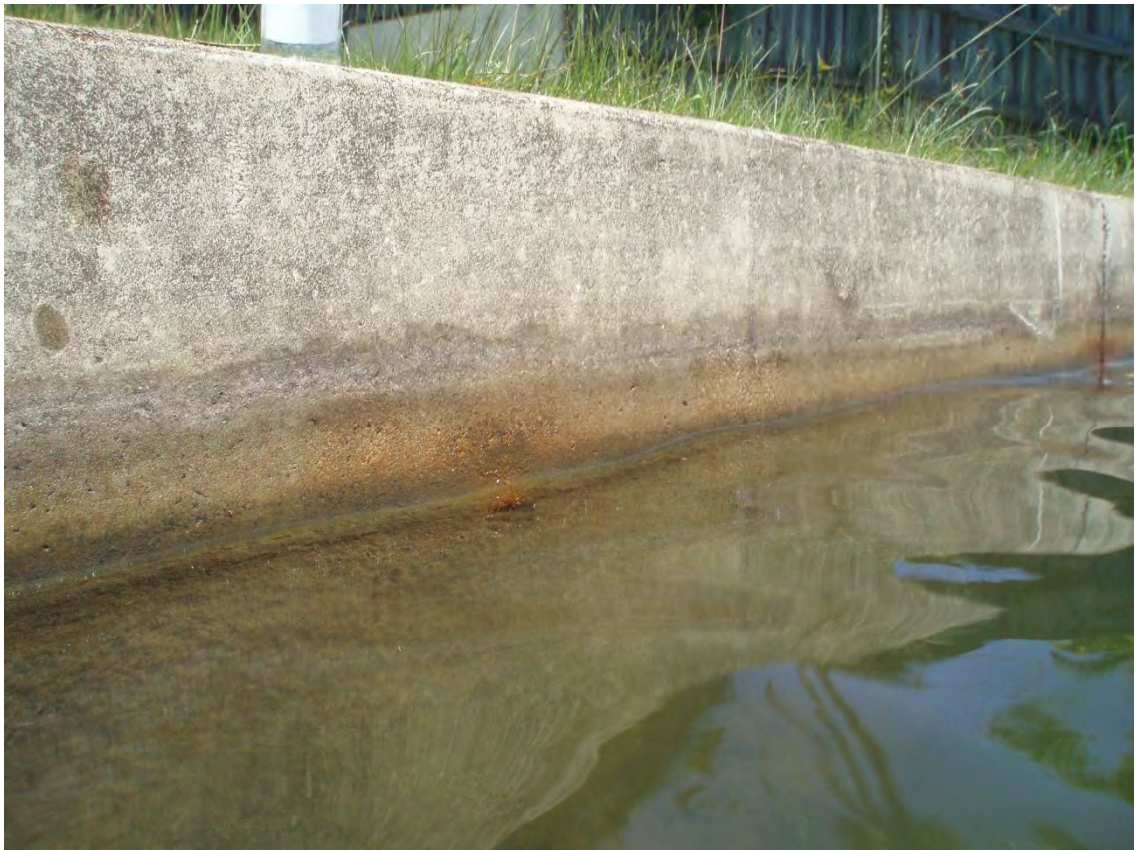
Figure 2-7 Wall sunken at 38 Saltwater Av, drainage holes are below water surface.
