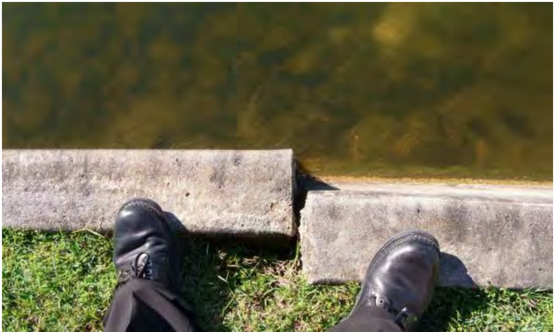
Figure 2-2 Revetment wall tilting forward at 37 Masthead Quay (SCRC 2012).
