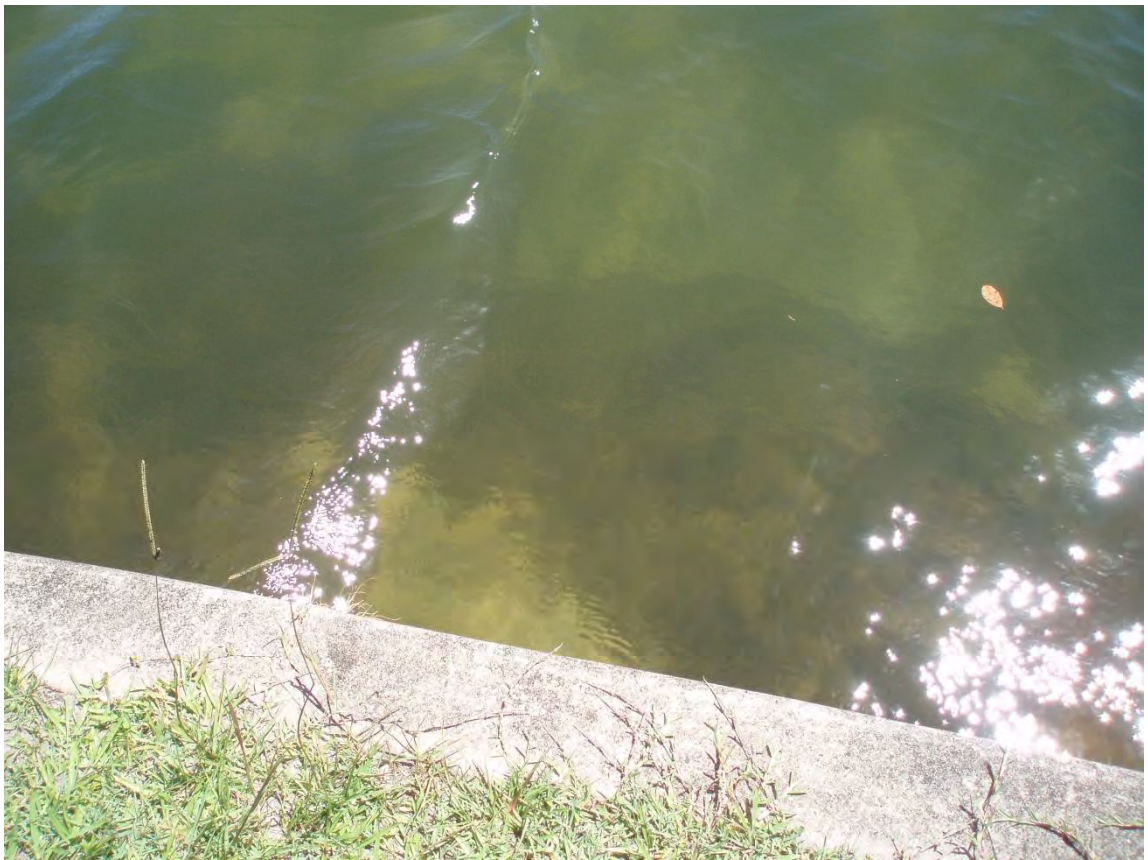
Figure 2-9 Section of scour protection moved slightly down toe.
