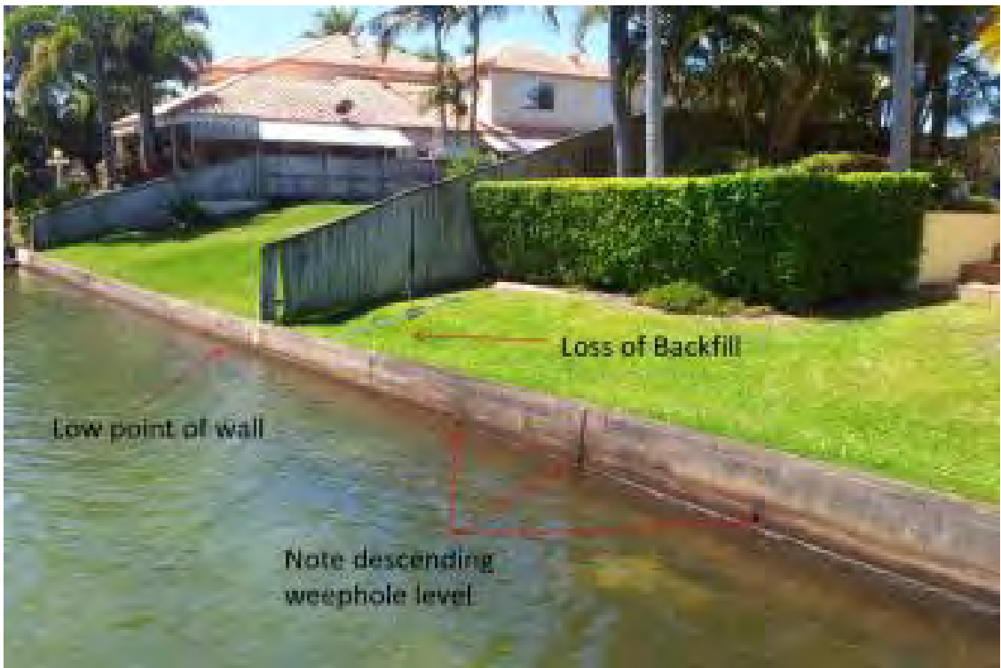
Figure 2-8 Sunken wall at 40 Saltwater Ave (Hall 2012).
