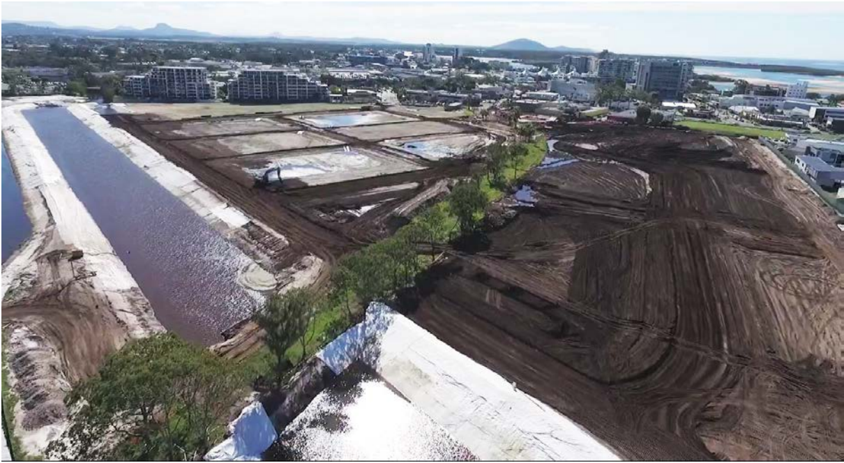
Image 1. North-west perspective: Corso waterway configured, establishment of city blocks/street network, existing 11KV protected corridor traversing the works area
