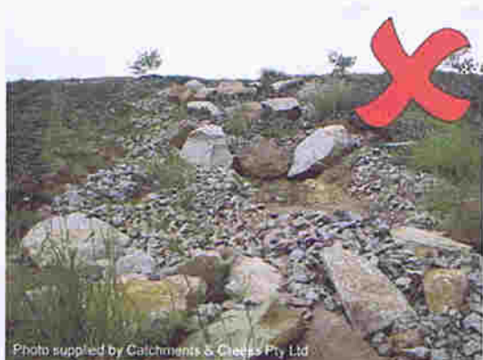
Photo 8 – Erosion caused by inadequate rock size and water bypassing around the poorly located boulders
