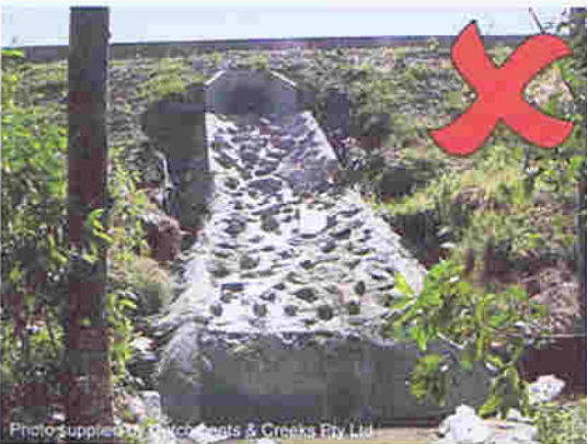
Photo 7 – Severe erosion along edge of chute caused by water spilling out of the chute
