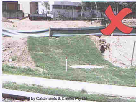
Photo 6 – Turf chute with poorly-defined inlet profile causing flow bypass
