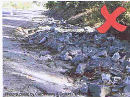
Photo 22 – In this example, placement of the rock has resulted in the rock-lined table drain being higher than the road shoulder
