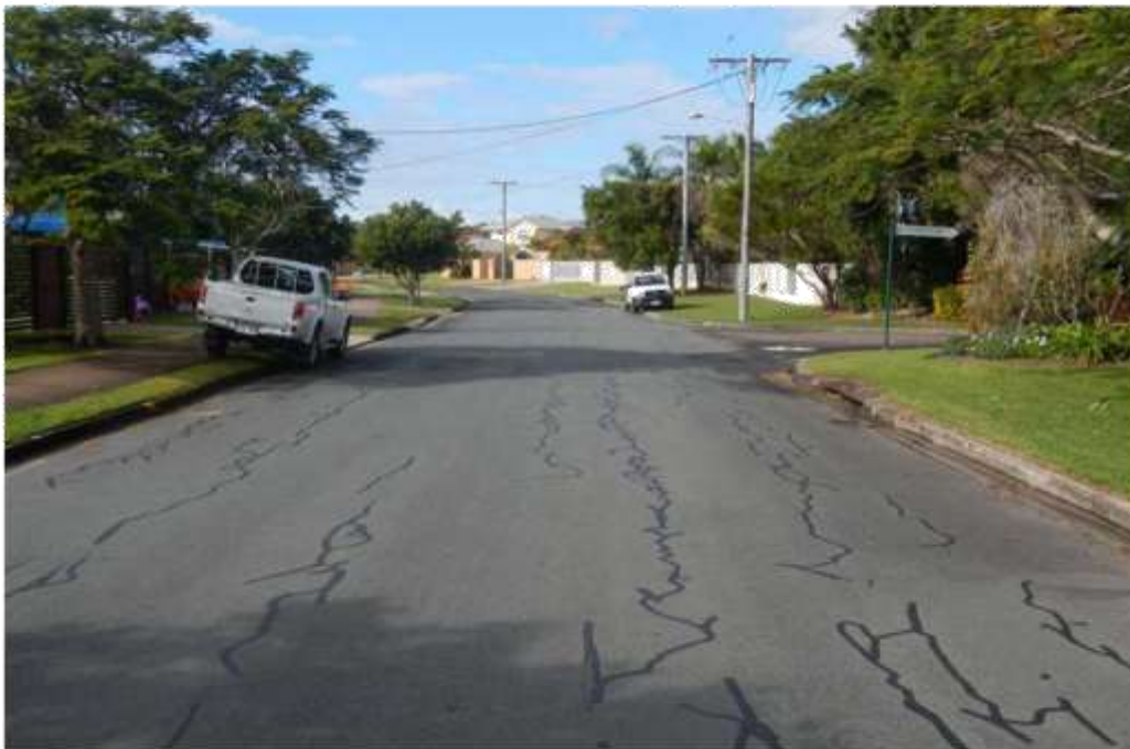
Photograph 10: View looking south along Lamerough Parade approaching the intersection with Cowiebank Place.
