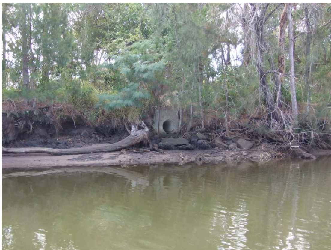
Figure 22: Stormwater drain near sampling site 3
