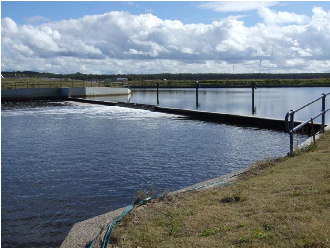
Figure 16: Weir between Lake Kawana (distant) and Lake Currimundi System (foreground)
