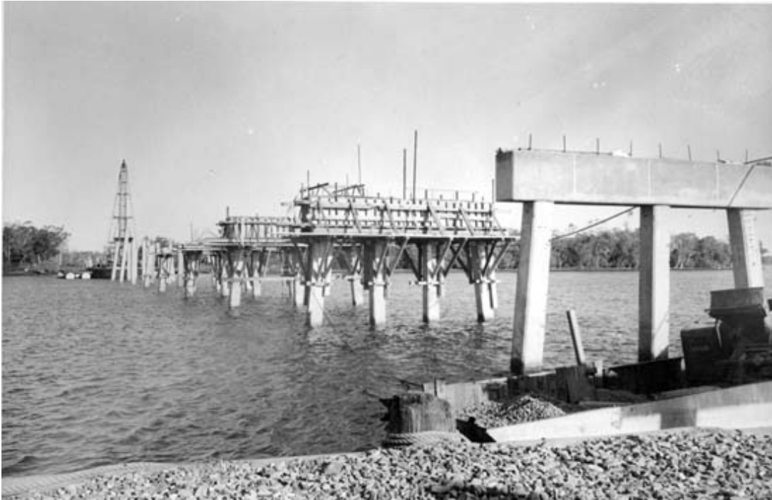
Figure 41: David Low Bridge under construction at Bli Bli, January 1958 (Sunshine Coast Library).
