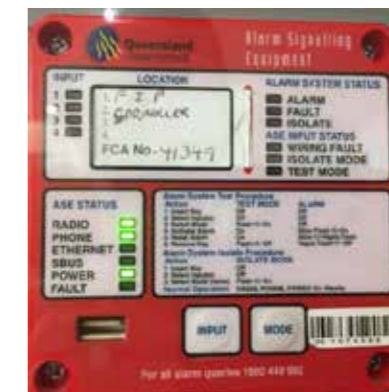
Figure 19 - Alarm Signalling Equipment indicating both Phone and Radio Connectivity
