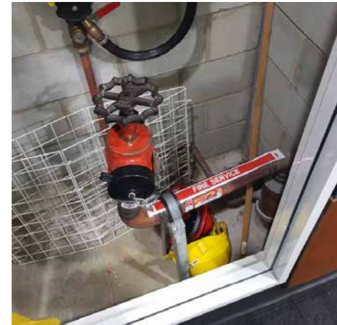
Fire Hydrant Cupboard Pipework
