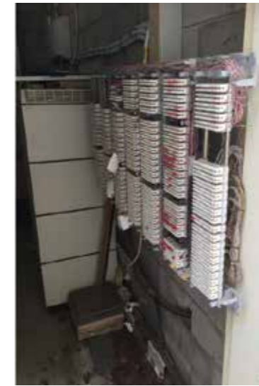
Figure 15 - Site Main Distribution Frame within Main Switchroom
