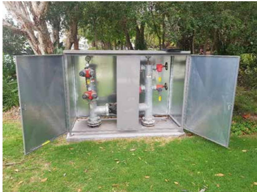
Existing Combined Site Hydrant Booster
