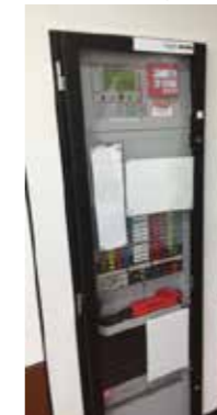
Figure 18 - Building Fire Indicator Panel
