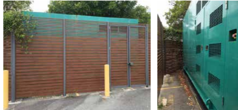
Figure 8 - Existing Generator Enclosure
