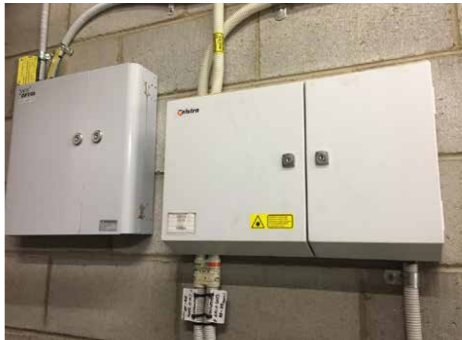
Figure 14 - Optus (left) and Telstra Fibre Lead in termination points
