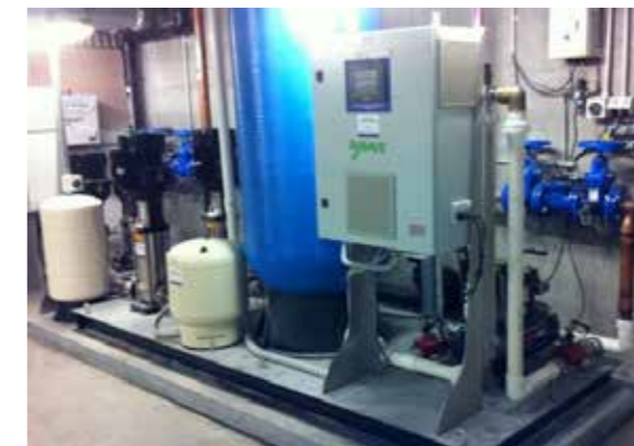
Typical Rain Water Plant
