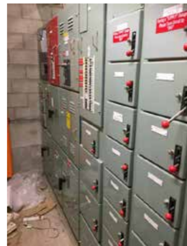
Figure 5 - Existing Site Main Switchboard
