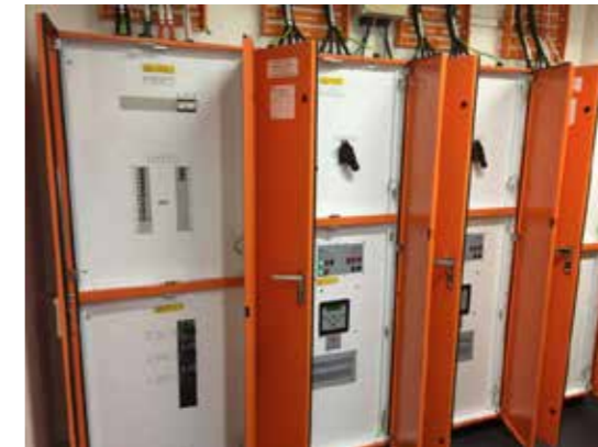
Figure 10 - Data Centre Main Switchboards A (left) and B (right)
