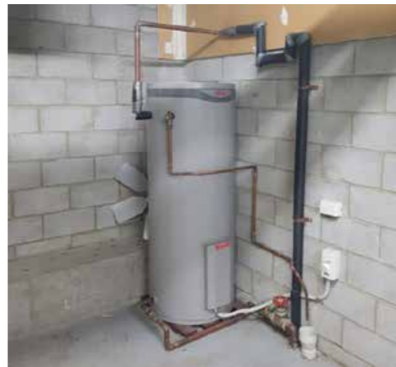
Storage Hot Water Unit
