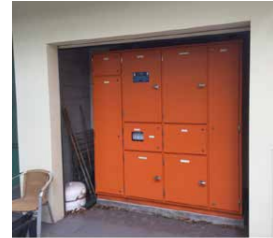
Figure 9 - Level 1 Generator Switchboard Accessed via Roller Shutter
