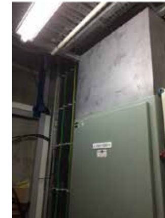
Figure 6 - Typical Distribution Board in Riser Space
