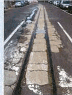
Mill Street, west of Currie Street showing broken concrete surround.
