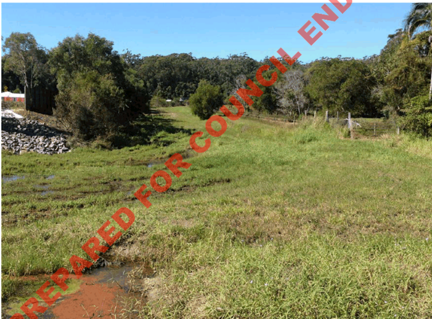
Figure 12 Poor Open Channel –Ponding, odour, weed incursion, unable to be maintained (source: Switchback Consulting)
