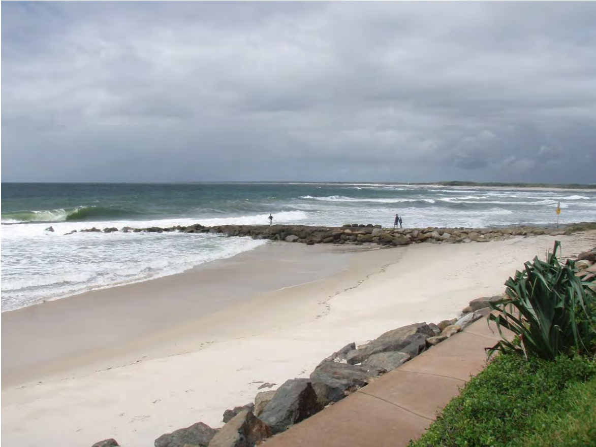
Figure 6.26: Photo of the existing groyne at Kings Beach, looking towards Bribie Island
