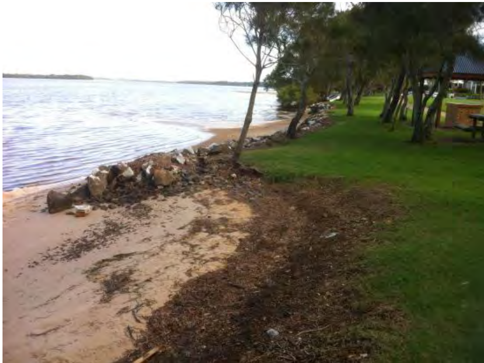
Figure 6.32: low revetment and adjacent erosion south of Lamerough Canal (EMC 2)
