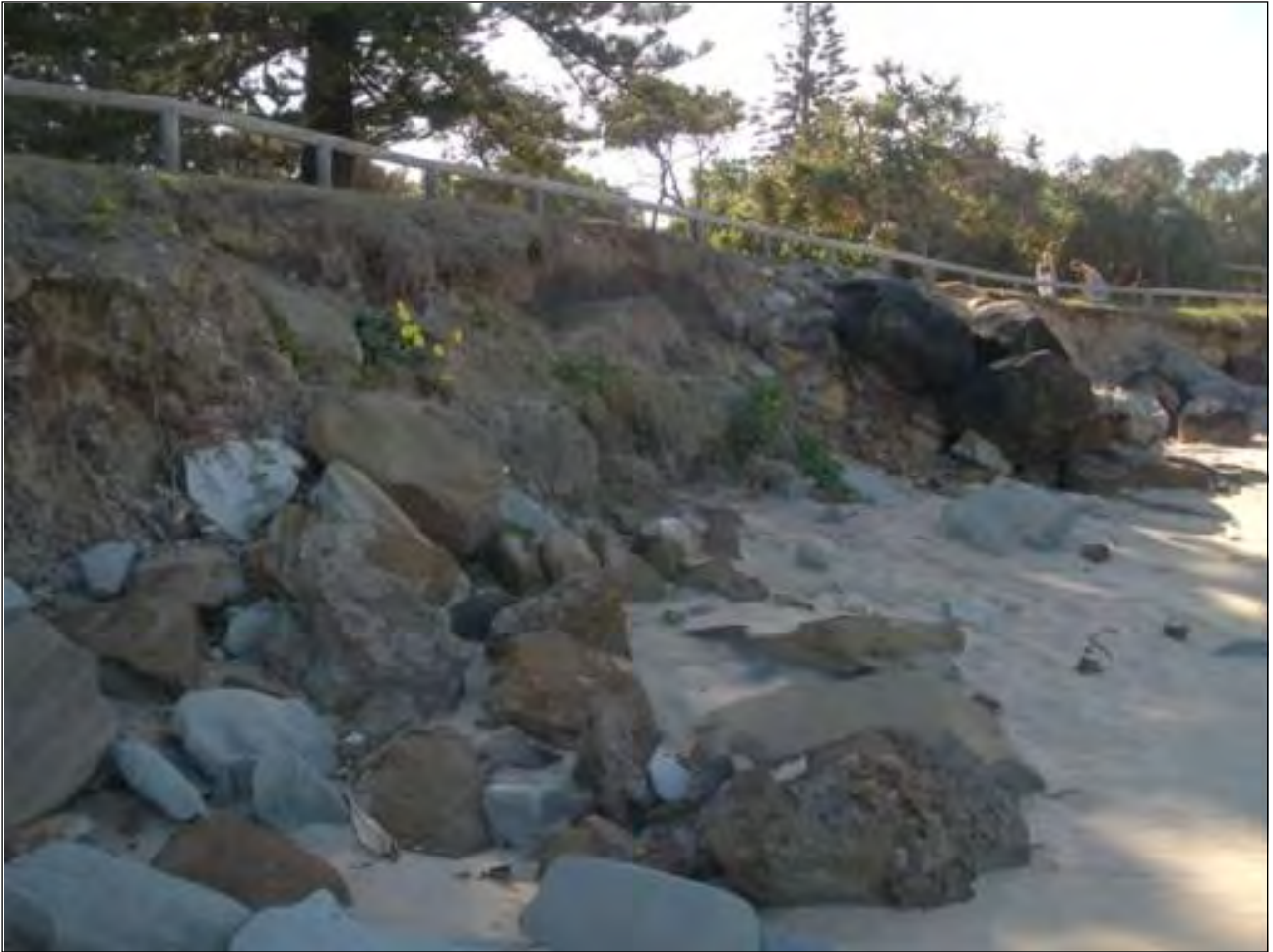
Figure 6.21: Degraded rock seawall protecting Lower Neill St car park, Dicky Beach
