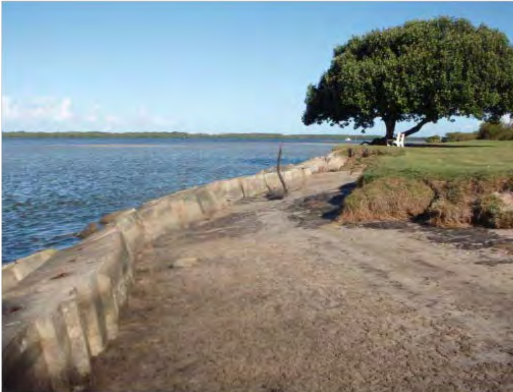
Figure 6.28: Photograph showing erosion behind concrete blocks placed at Navel Cadets Base (EMC 1)
