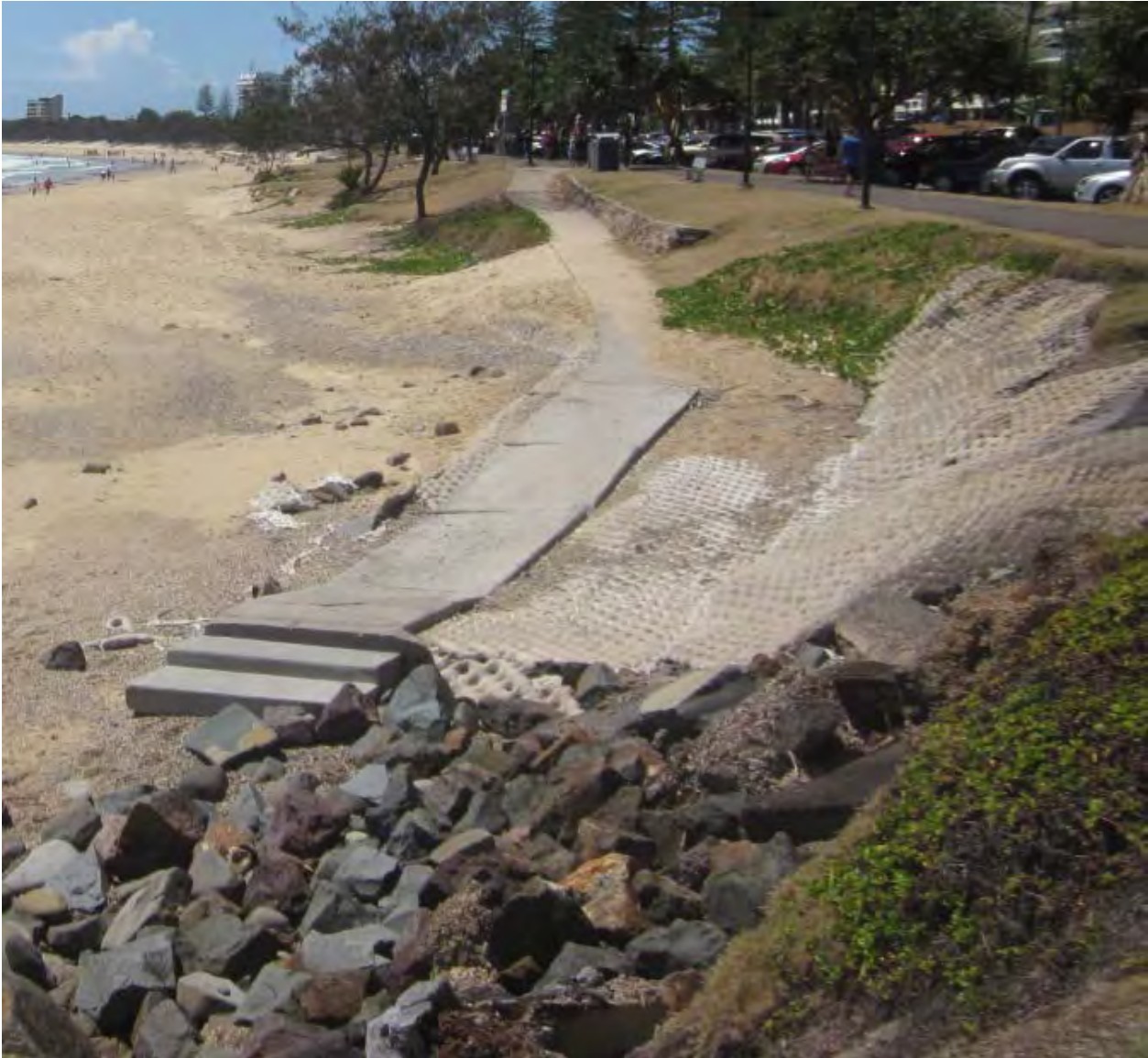
Figure 6.14: deteriorating rock seawall and light geo-formed concrete armoring at Mooloolaba Beach North
