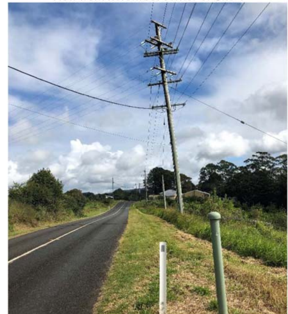
View of Energex poles through North Maleny Road
