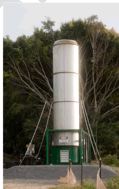
Image 16: Caloundra landfill gas flare
