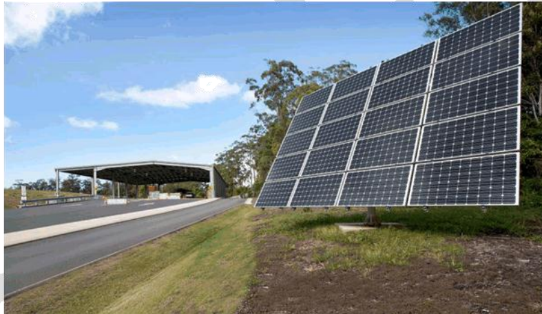
Image 13: Buderim resource recovery centre solar panels offsetting the sites power usage
