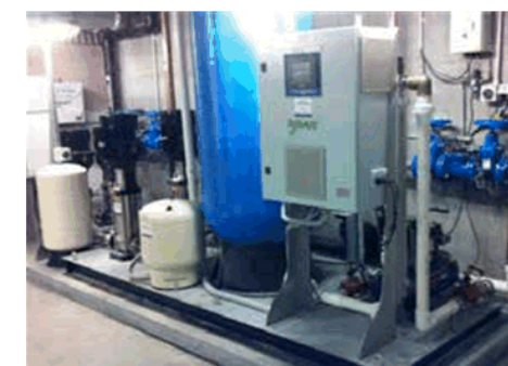
Typical Rain Water Plant
