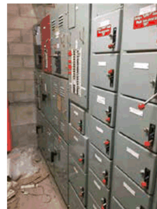
Figure 5 - Existing Site Main Switchboard
