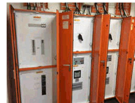
Figure 10 - Data Centre Main Switchboards A (left) and B (right)
