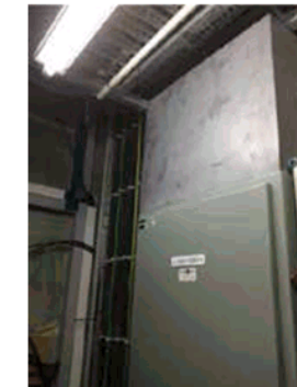
Figure 6 - Typical Distribution Board in Riser Space
