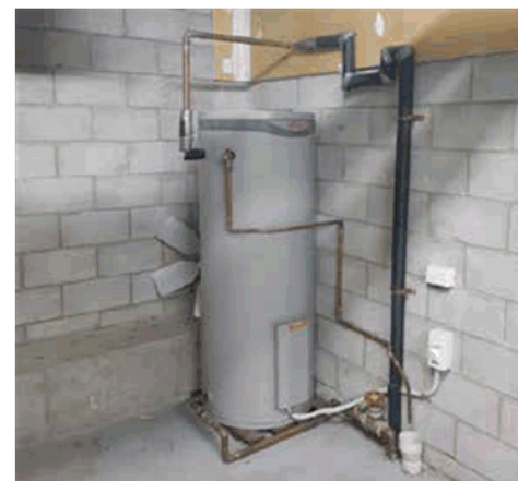
Storage Hot Water Unit
