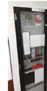
Figure 18 - Building Fire Indicator Panel
