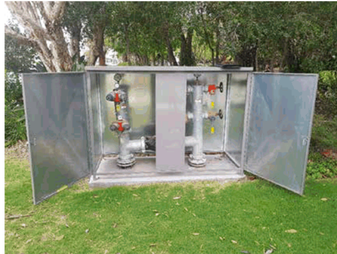
Existing Combined Site Hydrant Booster
