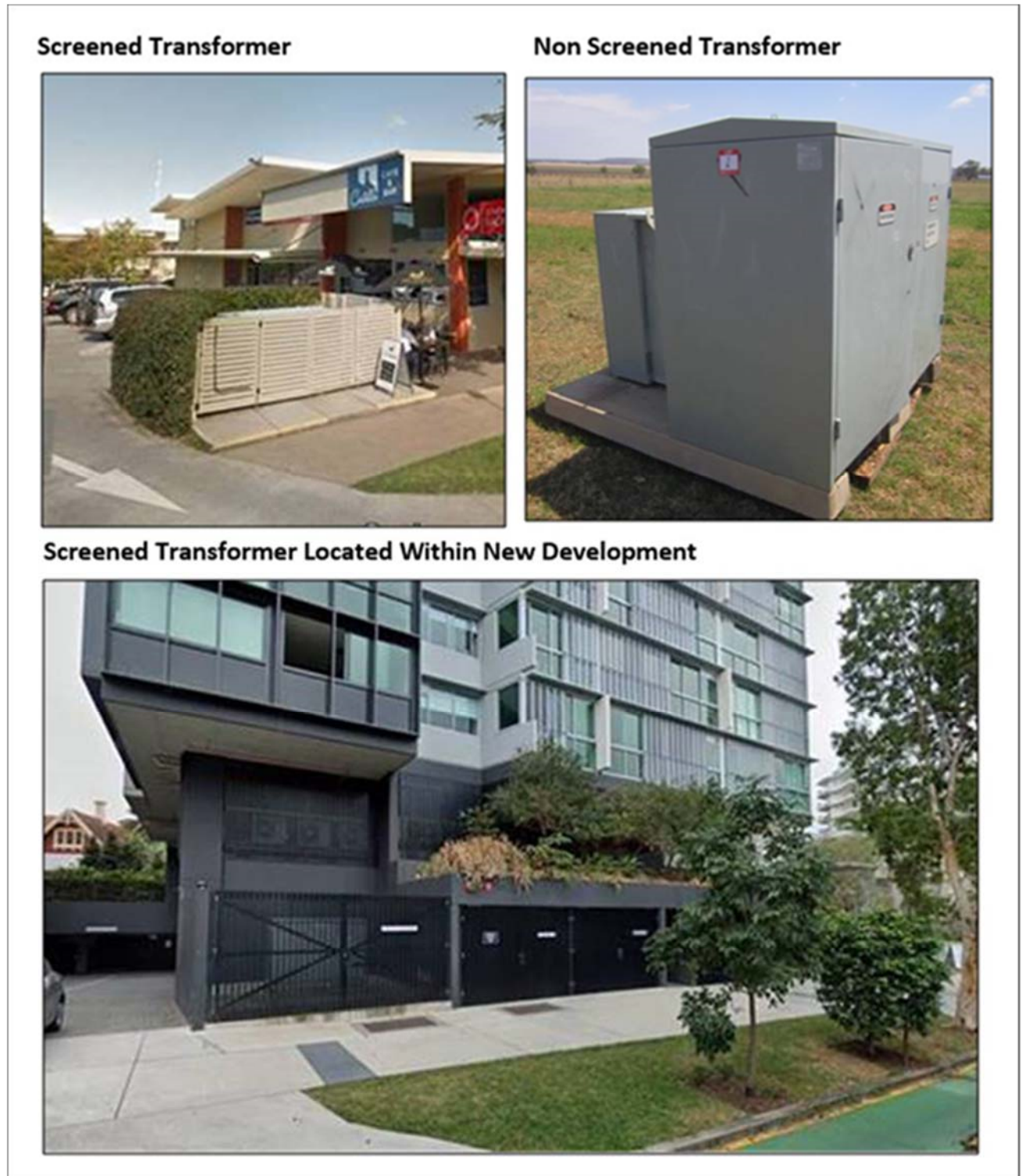
Figure 2 – Examples of Screened and Non-Screened Transformers
