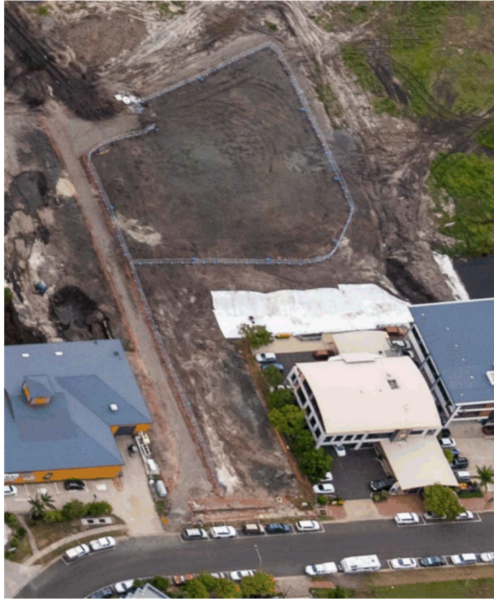
Stage 1A1 – Automated waste collection system transfer station site civil works (off Carnaby St)
