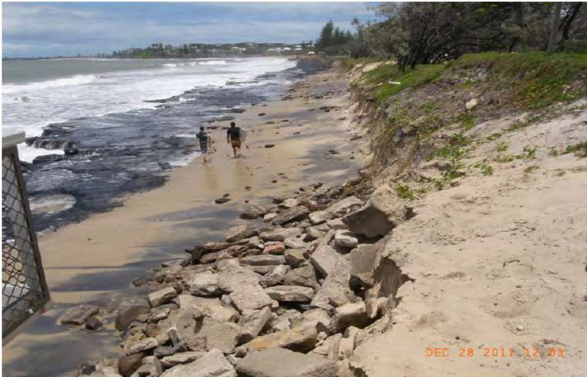
Photo 3 – Exposed beach fill north of Alexandra Headland Surf Life Saving Club, Dec 2011
