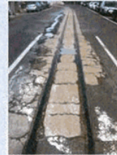
Mill Street, west of Currie Street showing broken concrete surround. ¶
