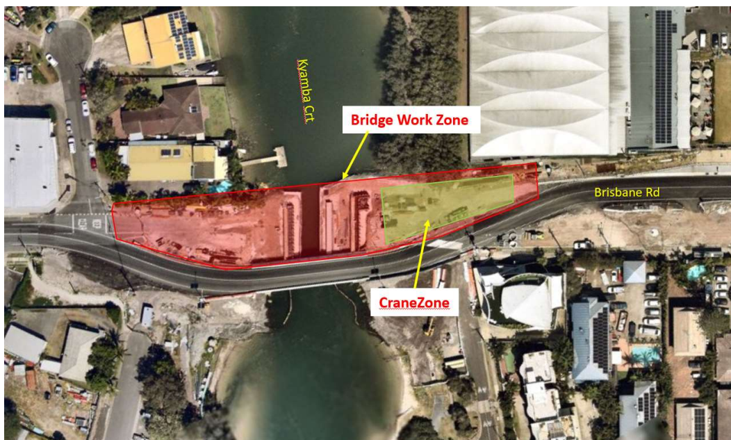
Figure 1. Crane location and western lanes of new Mayes Canal Bridge currently under construction – Brisbane Road *all works are weather and site conditions permitting.
