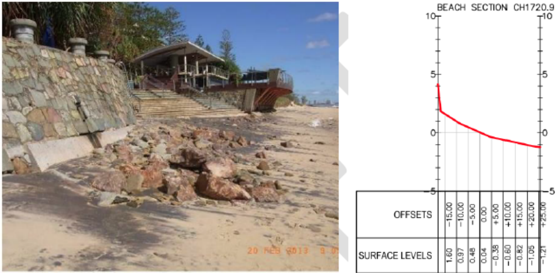
Figure 5.3 Present seawall following TC Oswald 2013
