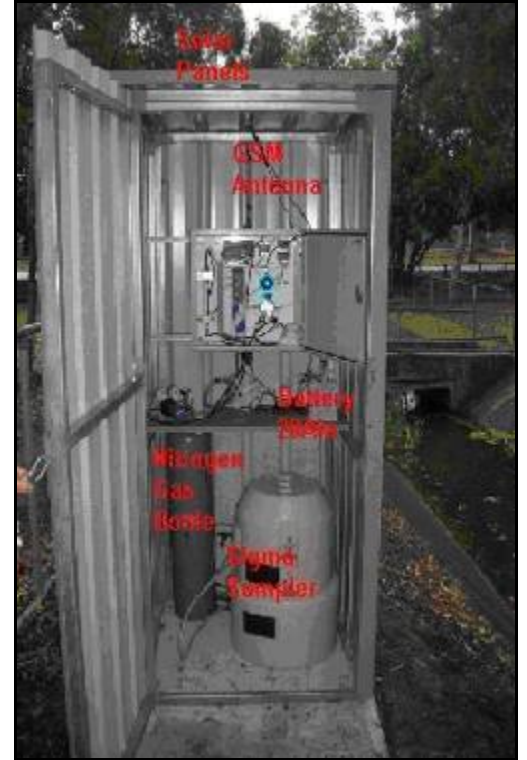
Typical Enclosure Contents
