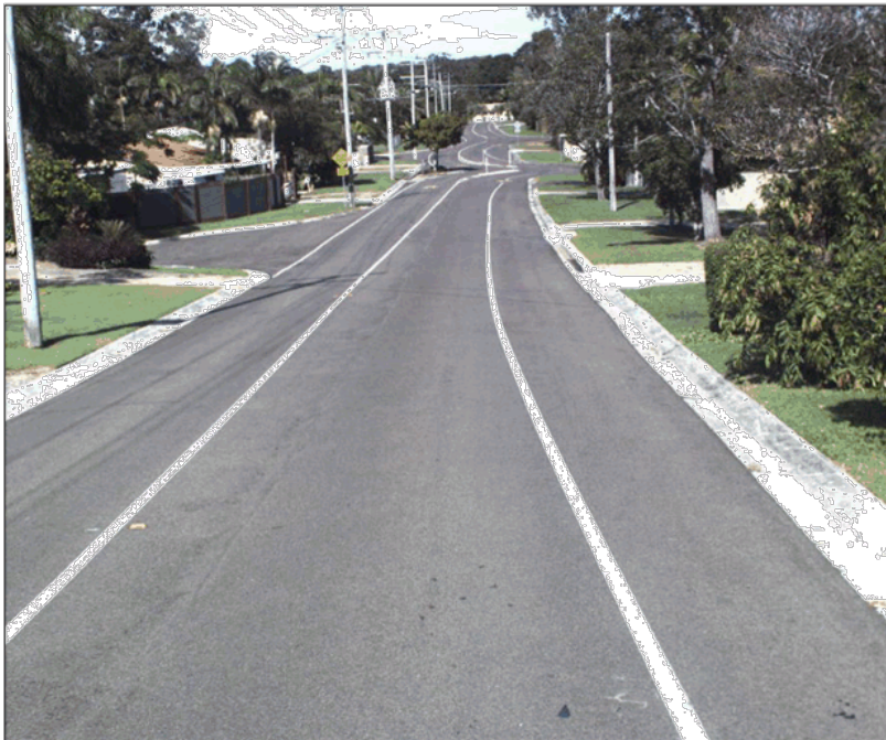
Figure 4: Pavement Condition Index 8
