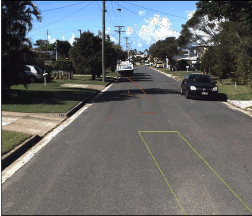
Figure 3: Pavement Condition Index 7
