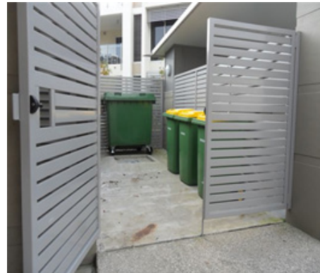
Screened waste storage container area with bunded bin wash down area.
