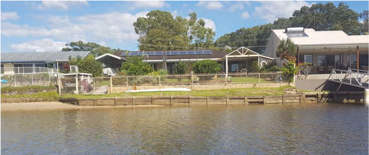
Figure 3-5 Grass stabilised canal beach with unapproved timber revetment wall
