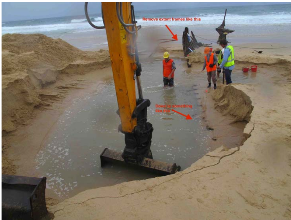
Figure 43. Example of where frames are to be cut down to on starboard side. The stubs in the foreground are the tips of the floors, the frames having been removed by recent storm surges. (Cosmos Archaeology, 28 April, 2014)
