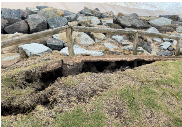
Seawall reconstruction: A section of the seawall collapsed due to soil failure, necessitating reconstruction which meets engineering standards.
